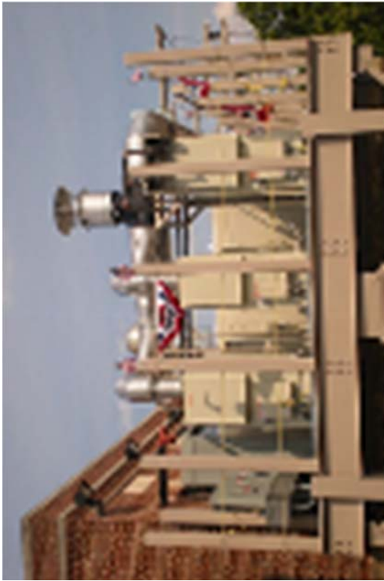
360kW CCHP Microturbine/Chiller Plant at Windham Community Hospital, CT
